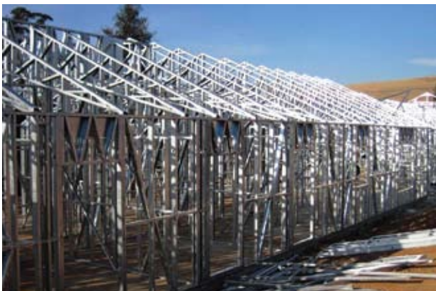
LSF construction in progress on the nurses' accommodation block at the St Apollinaris Hospital in KZN
