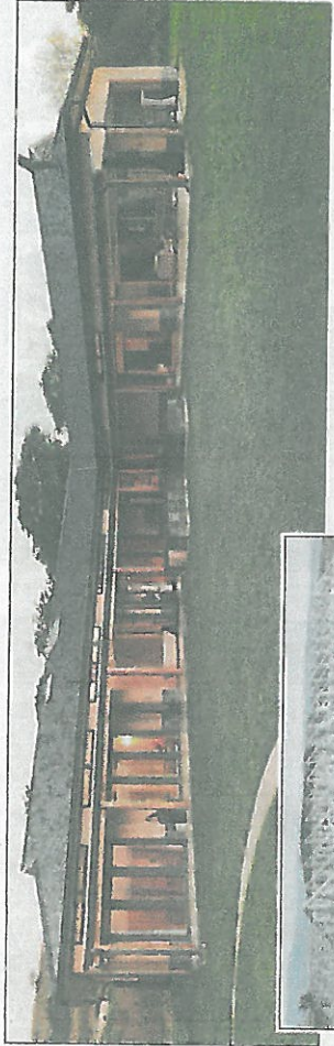
Left: The light steel structure of this home in Pietermaritzburg was erected in just a few weeks. Above: The completed house, which has saved the owner in energy costs because of the thermal design.
